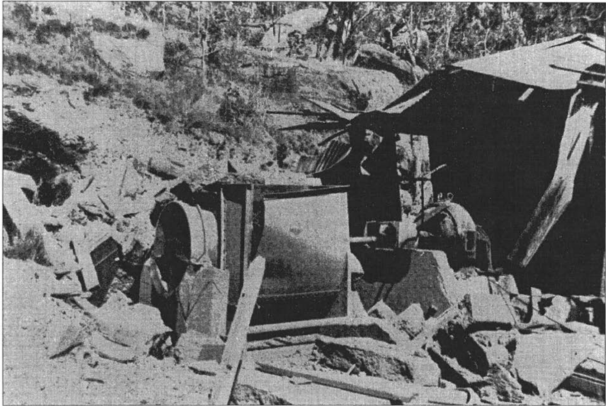
16. Ventilating Fan Motor blown from the return airway (No.3 Adit) by the explosion
